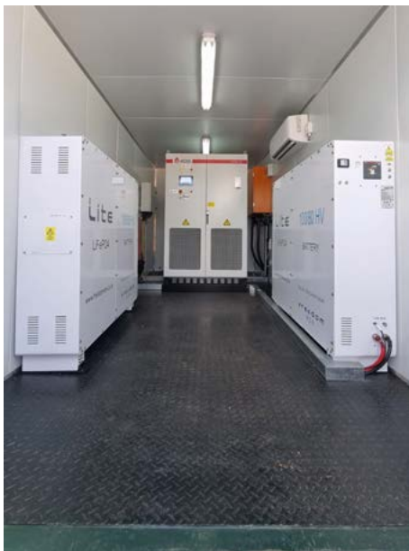
Air conditioned solar control room, in a reconditioned container.
